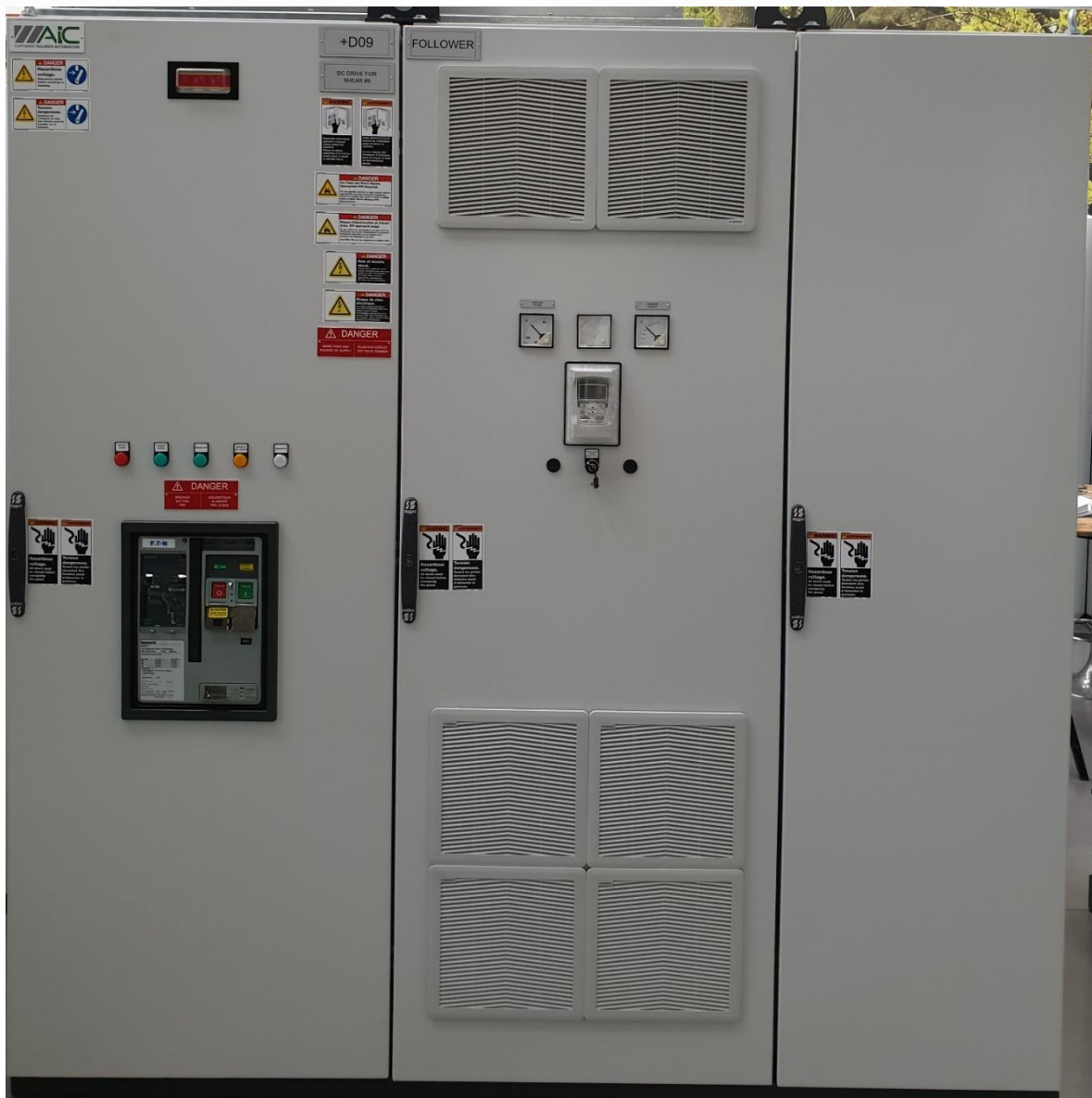
(one of the previously supplied drives to site)
