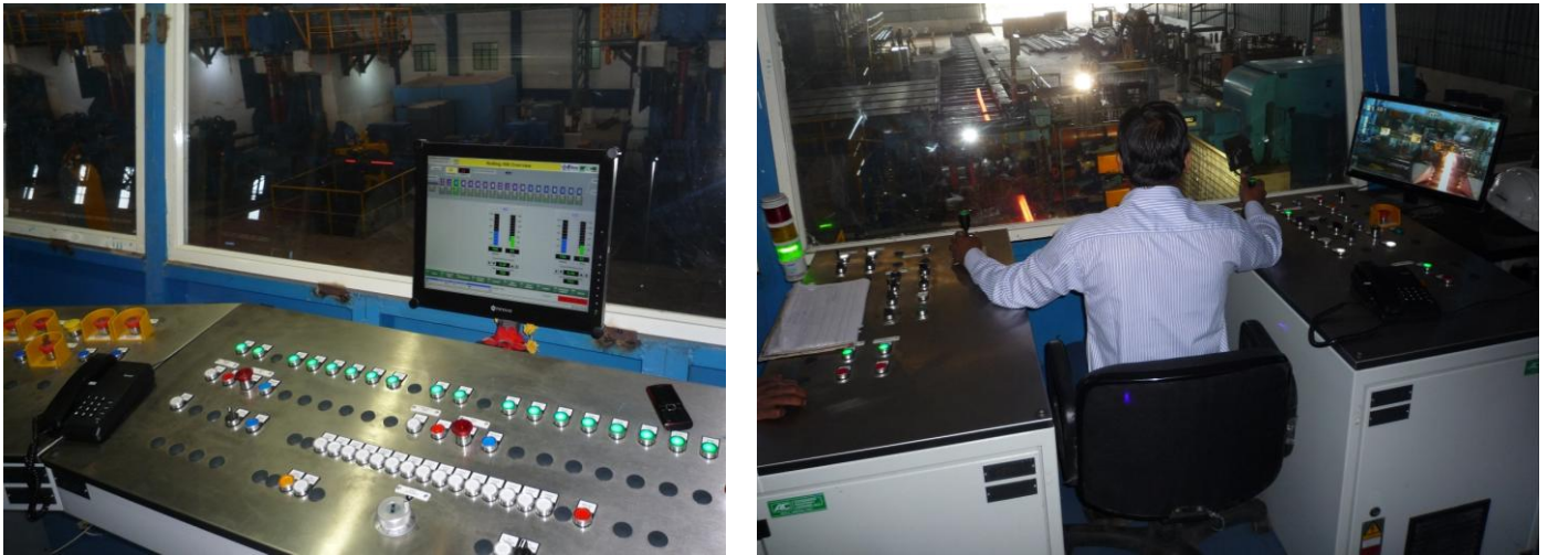
Fig. 4-5: Main control desk and local roughing mill pulpit
