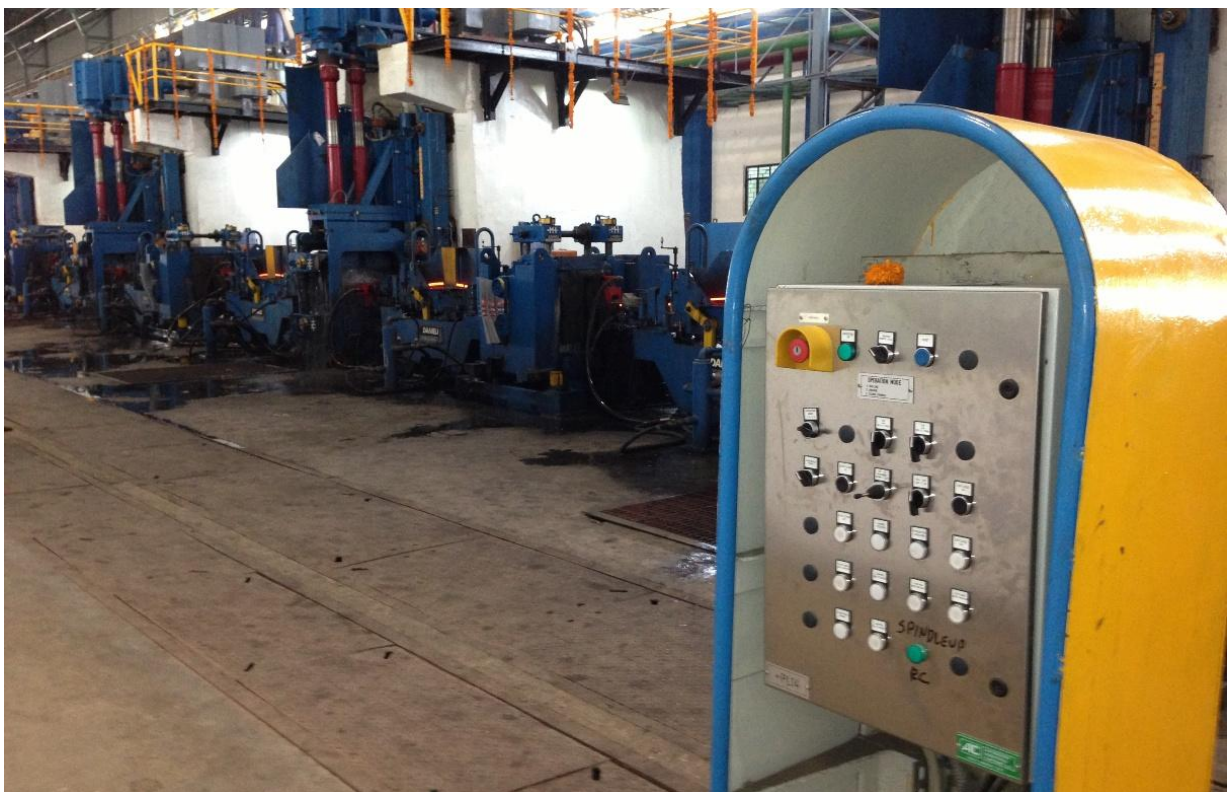
Fig. 1: Rolling mill and AIC local control station
