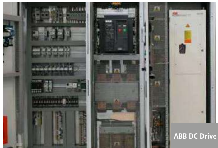
4 Main DC Drives Panel for Blooming Mill control with Nidec-Ansaldo
