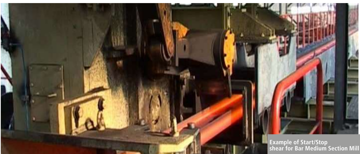
Example of Start/Stop shear for Bar Rolling Mill
