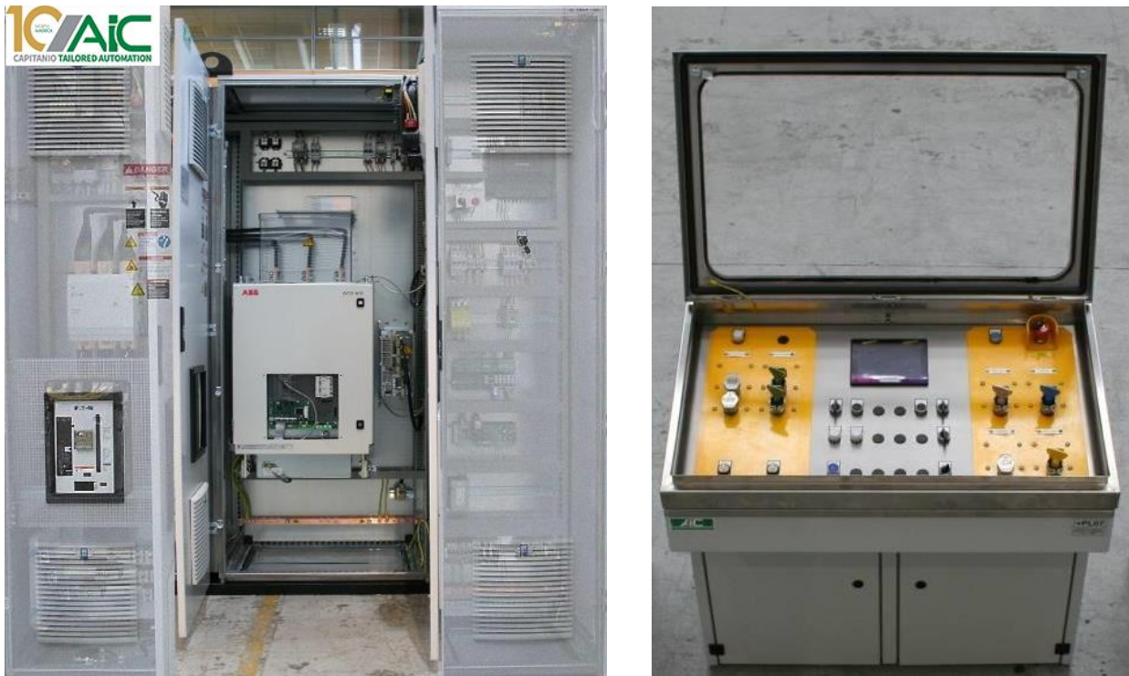
Figure 1 – Example of Main DC Drive Panel manufactured by AIC with DCS Converters and local control desk with safety functions.
