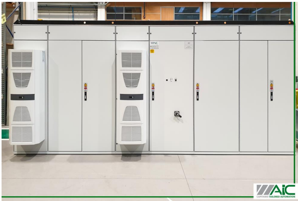
Fig. 1 – Control panel installed at the beginning of 2020
