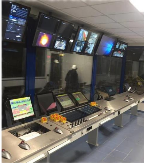
The example of the main pulpit for the control of the rolling mill
